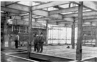
Figure 49. Construction of the Security Warehouse, 1954, showing erection of the steel posts and beams (Two Centuries of Corrections).
