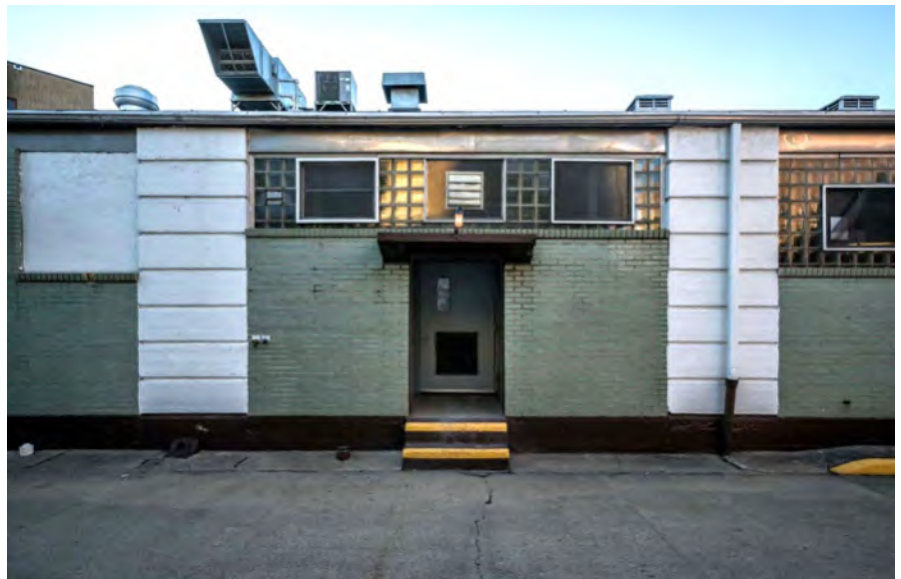
Photo 53. Dining Hall, east facade, looking west, showing a side entrance and typical building materials, such as mint green glazed brick, painted concrete piers and glass block.
