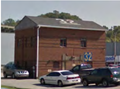
Figure 6. Maintenance Storage Building (32), looking east, showing typical building designations used on walls and roofs (Google).
