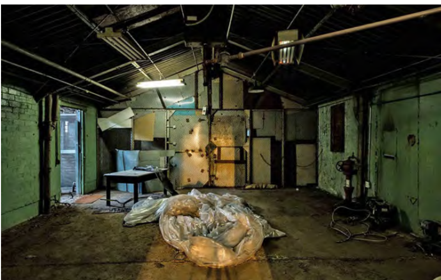
Photo 51. Correctional Industries Shop Building interior, infill connector between the Tag and Metal Shops, looking west. The electrical substation is beyond the end wall.
