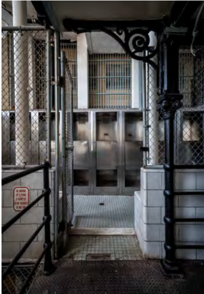
Photo 19. Main Penitentiary Building interior, Housing Unit D, looking north, showing typical stainless steel shower units.
