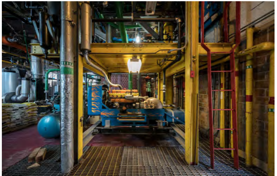
Photo 80. Boiler Plant interior, looking north.
