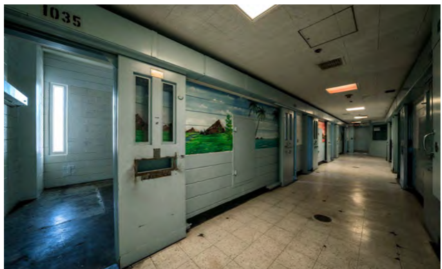
Photo 77. Health Services Building interior, first floor, looking northeast, showing a typical corridor (right) and patient cell (left) with its narrow window.
