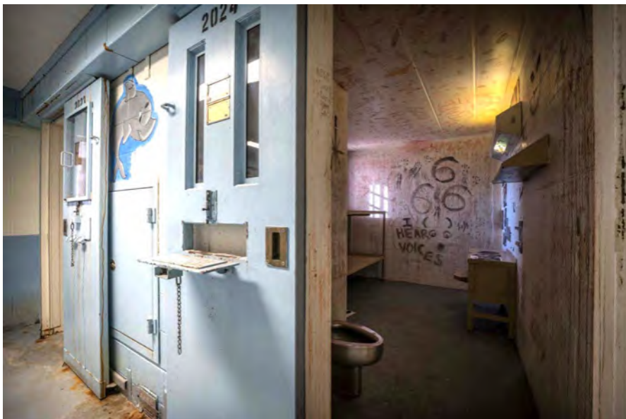
Photo 32. Housing Unit A/Building 5 interior, showing a typical second floor corridor with sliding doors and the inside of a typical cell. The fold-down panel in the center of the door was a safety feature. With the inmate inside the cell and the door locked, the inmate would place his arms through the opening. Guards could then safely attach handcuffs before opening the door. This particular unit retains considerable graffiti from its last inmate in 2017.
