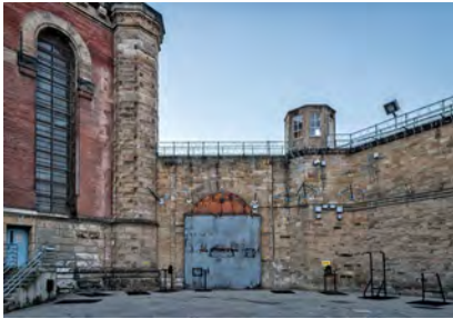
Photo 87. Northwest gate (no longer in use), looking west from within the Secure Perimeter, showing Tower 1 atop the wall.
