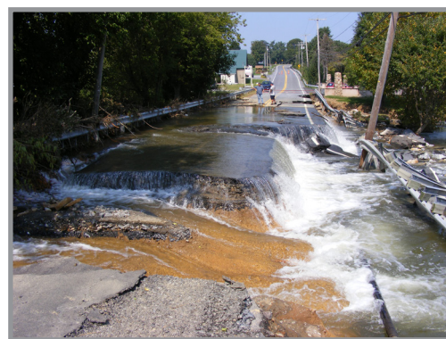
Flood damage requires emergency repairs
