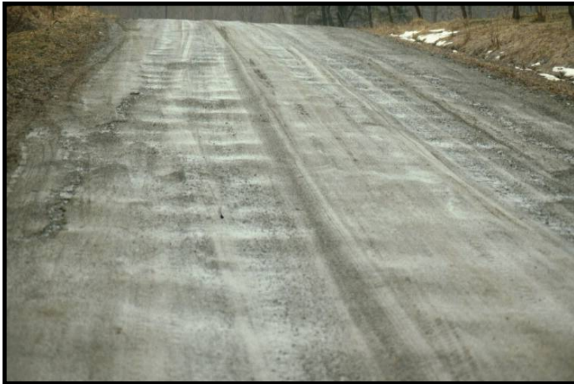
Corrugations - Low Severity
