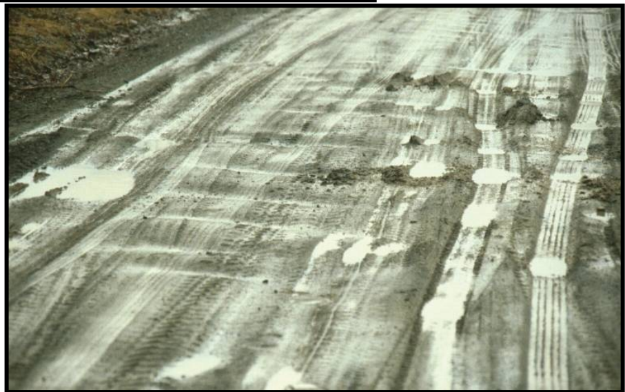
Corrugations – Medium Severity
