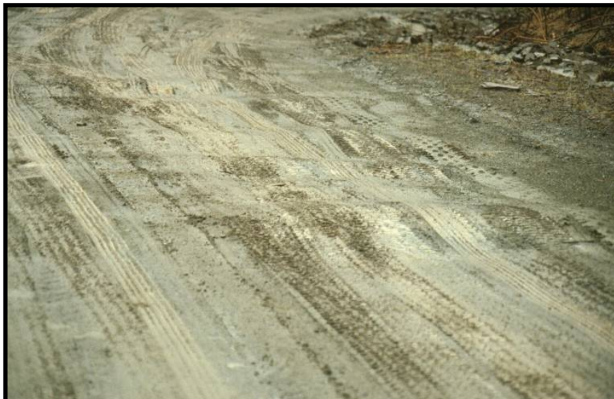
Corrugations – High Severity
