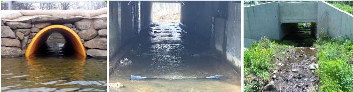
Examples of culverts designed to allow aquatic wildlife
