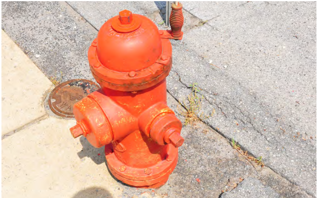
Fire suppression systems exist in parts of the corridor, but are not yet combined in a complete loop
