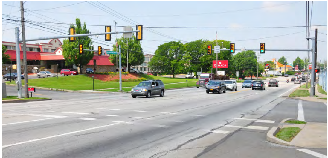
Faded pedestrian crosswalks at the Dutch Wonderland entrance
