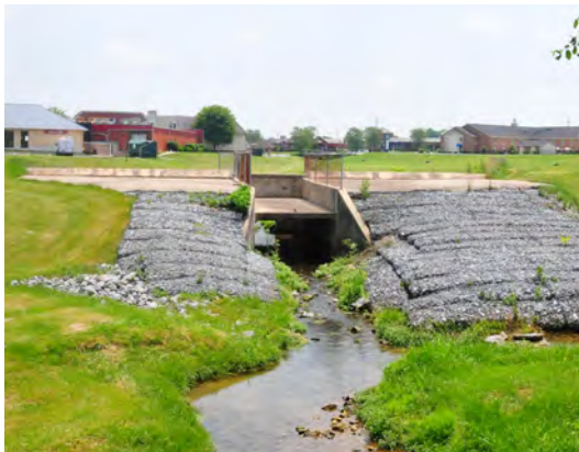
Stormwater device at Rockvale Outlet
